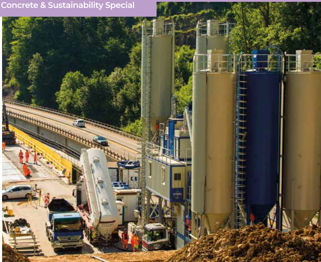
Fibre-reinforced high performance concrete was lately used on three bridges along the A4 Küssnacht-Brunnen motorway.
