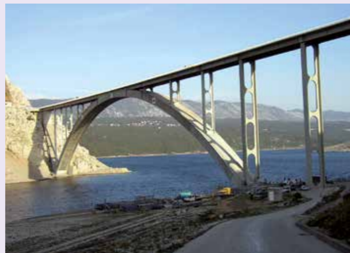
Structures with high mechanical properties are constructed thanks to concrete, such as the bridge on the island of Krk in Croatia.
