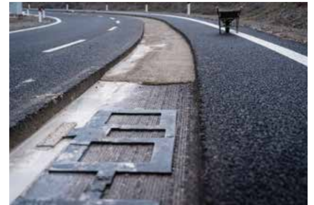
Mapei products were used to make the road layers housing the magnetic coils that allow wireless charging.
